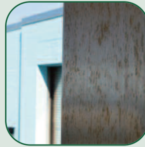
Staining from iron contamination Salt / chlorides present
