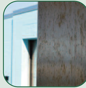
Staining from iron contamination Salt / chlorides present
